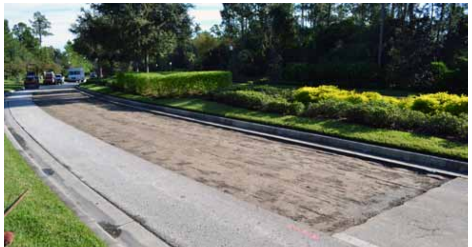
Repairs to an area of Ancient Oaks Blvd in front of Shoregrass on October 13, 2011.
