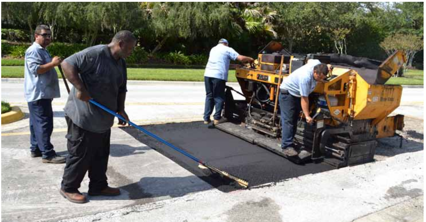
DuraSeal Asphalt Sealing and Paving Company repairs an area of Ancient Oaks Blvd in front of Brookforest on October 8, 2011.
