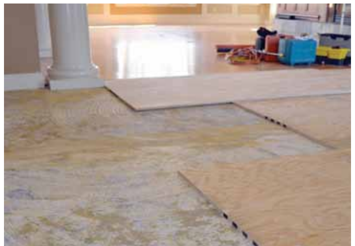
Plywood is being installed after carpet is removed from Gathering Room to bring this portion of the floor to the same level for tile installation.
