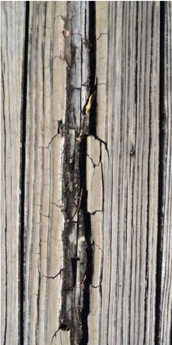
Rotten board on bridge on nature trail.
