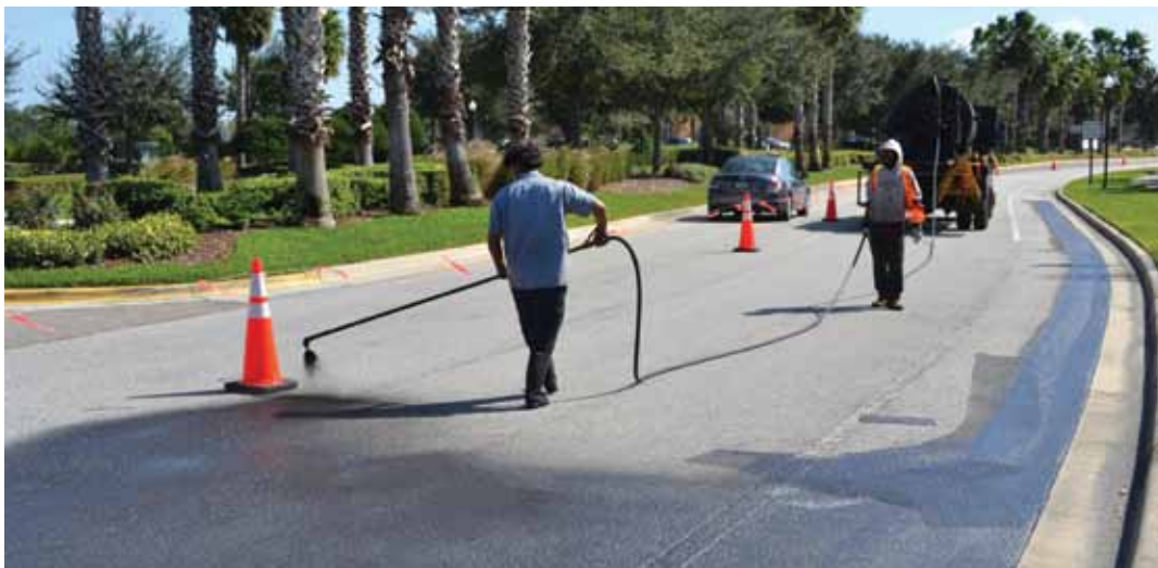
DuraSeal asphalt sealing and Paving put a seal coating on Ancient Oaks Blvd in November 2011
