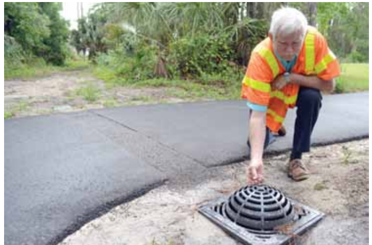
Jack engineered a drain system to keep the nature trail from flooding
