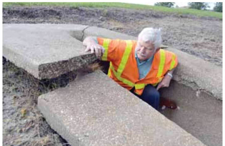
Jack inspects the pond drainage system that needs repairing
