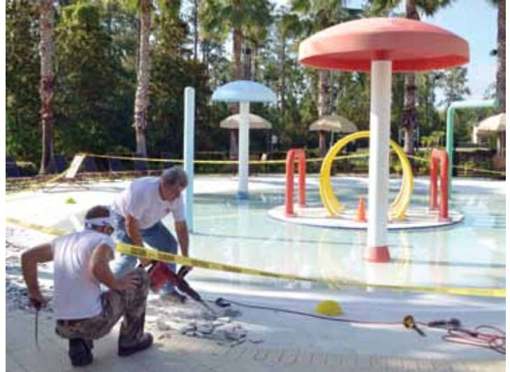
Speciality Services workers remove perimeter at the Splash Water Park. Aqua-Flex was chosen to replaced it (see picture below).
