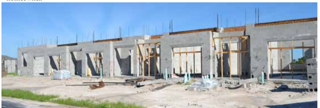
Start of construction of a row of eight D. R. Horton townhomes in Lakeside
