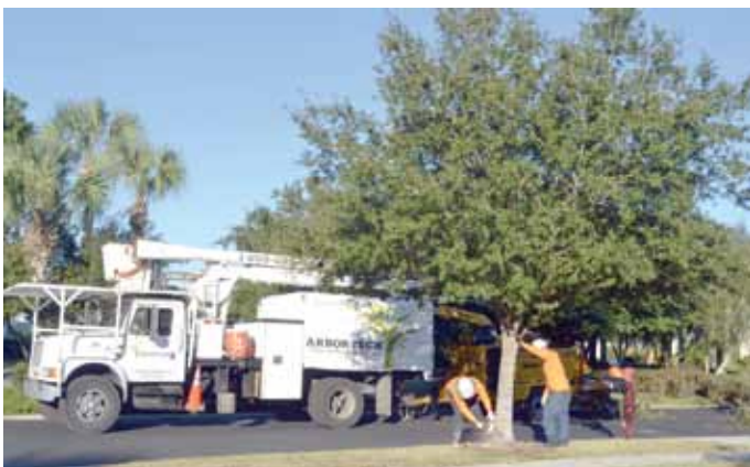
Arbor-Tech employees cut notch in the tree trunk prior to pushing it over.
