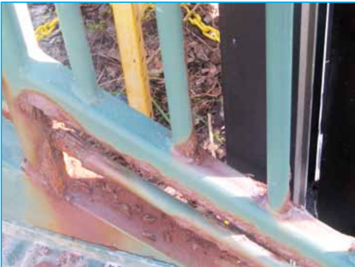
This is an example of how some of the railing rusted from the inside out and had to be replaced before it could be painted.
