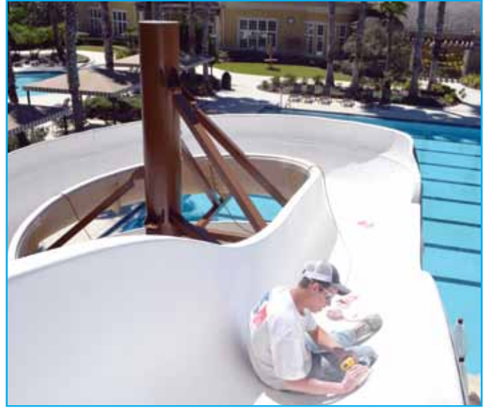
Derrick Bolding, Kalos Coatings employee, sanding the inside of the slide to make it smooth. It will also provide a faster ride.
