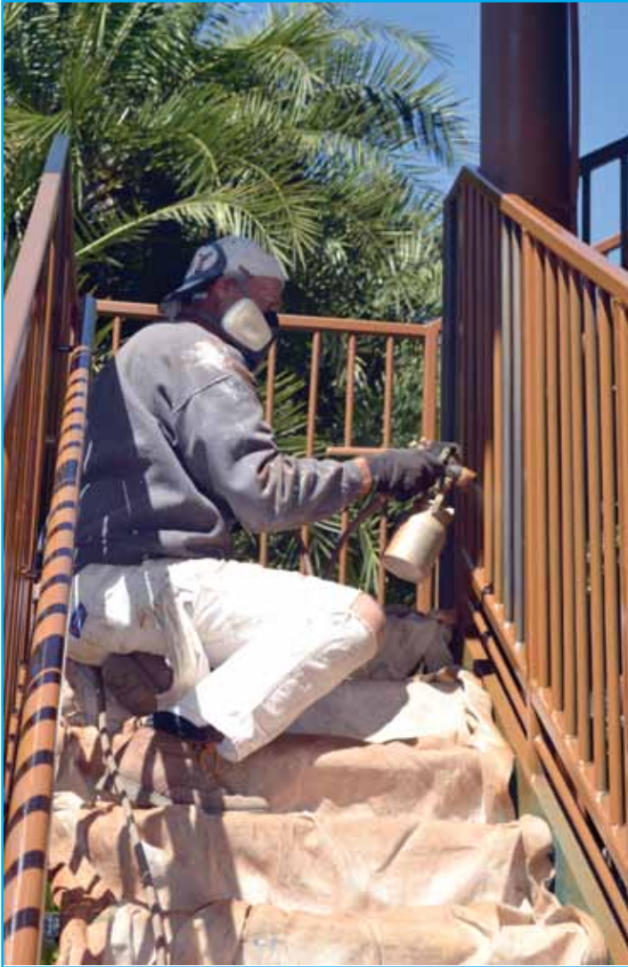
Steve Swartz, Kalos Coatings employee, sprays primer on the railing going to the top of the slide. Prior to putting on the primer, all rust was removed and any bad areas repaired.
