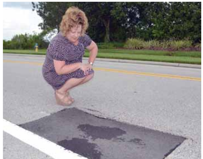
Tonja Stewart inspects an area of Ancient Oaks Blvd just south of Bellafield that has been repaired. One of the high priorities of Ms. Stewart is to insure that the roads are adequately maintained.
