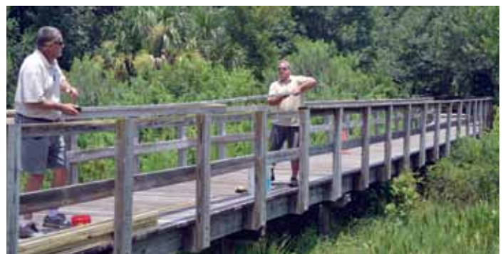
Bob and John repairing the bridge on the nature trail between Edenfield and Grassglen
