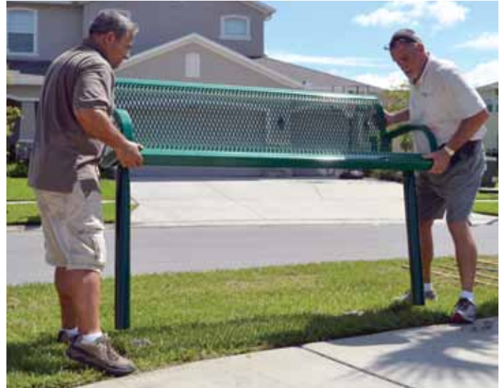
John Gentellella and Bob Semple install a bench in the Sable Point park.
