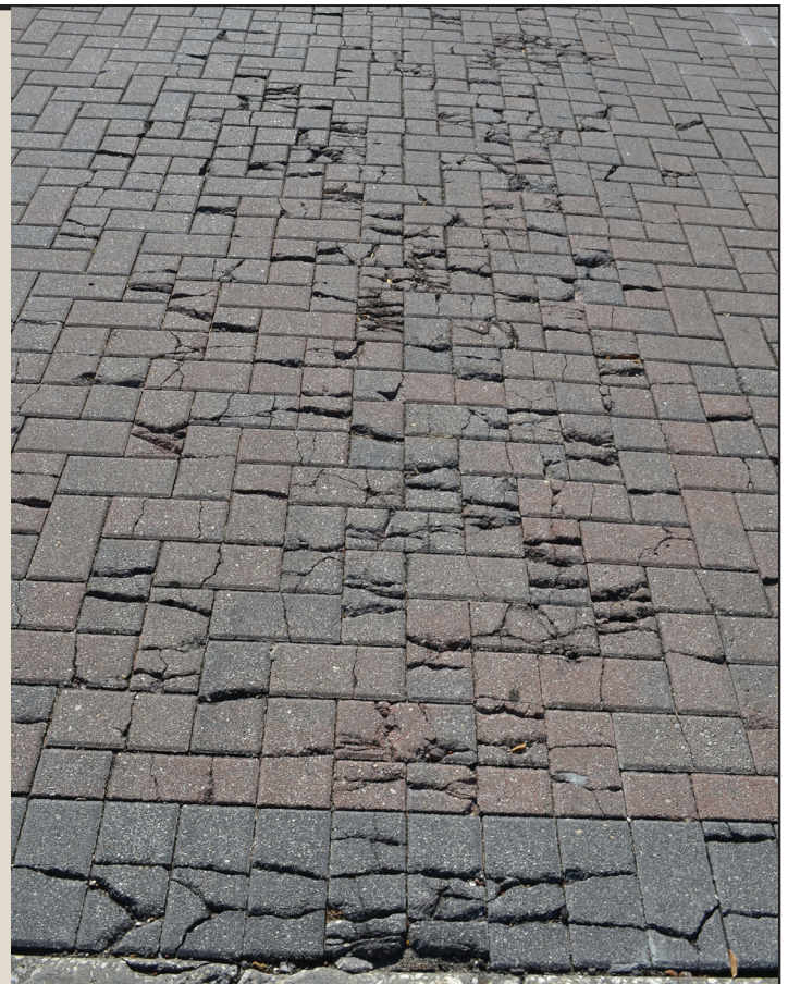
The above pavers at the north traffic circle have begun break up. These pavers and others at this traffic circle will be replace with asphalt.
