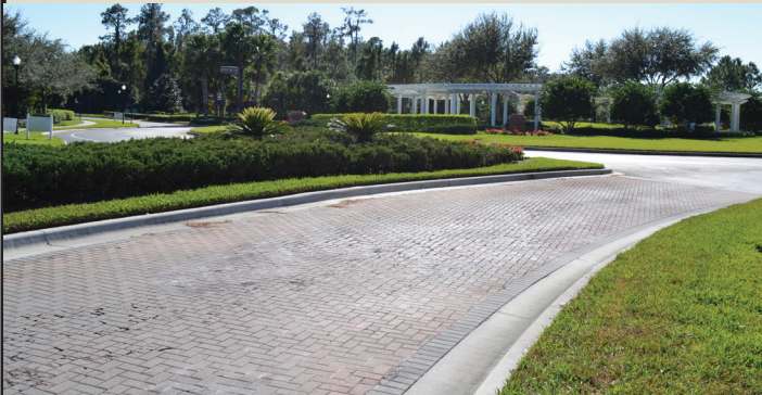
This is a view of the north traffic circle. At the bottom is the strip of pavers that have deteriorated the most
