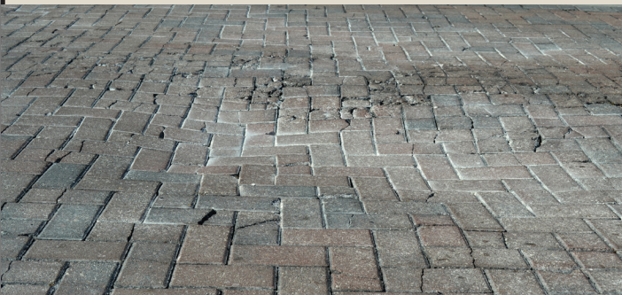
The above pavers are at the north traffic circle. This picture shows how some of them have sunk into the ground.
