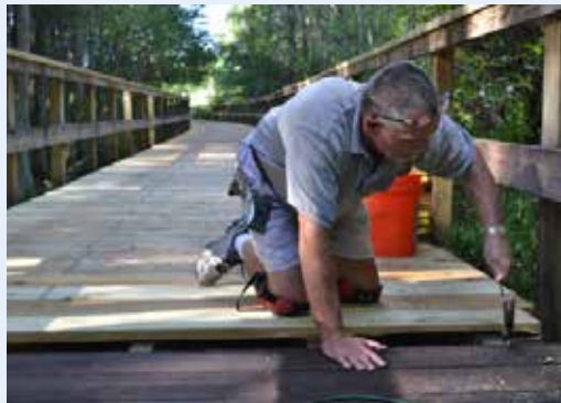
Bob Semple, Maint Superintendent, replacing boards on the bridge between Edenfield and Grassglen
