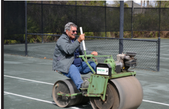
Larry Way uses a roller to insure nail heads are at tape surface
